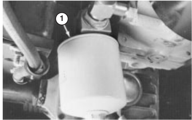
Figure 64 1. Hydraulic oil filter
