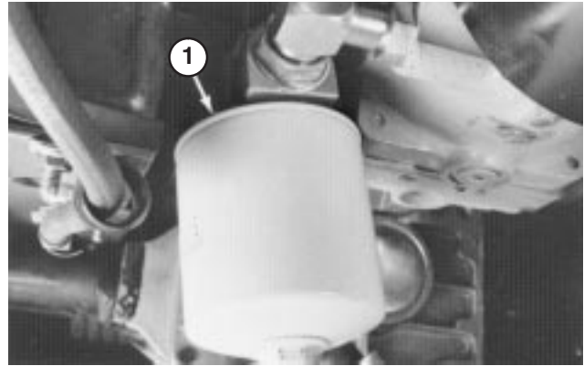
Figure 64 1. Hydraulic oil filter
